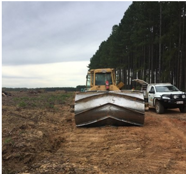
Figure 1. Chopper roller for site preparation - breaks down larger debris prior to planting, maximising debris retention.
