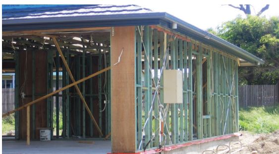
Figure 2 Termite management for this house includes concrete slab physical barrier coupled with chemically impregnated plastic perimeter and penetration barriers and termite treated wall and roof framing.
