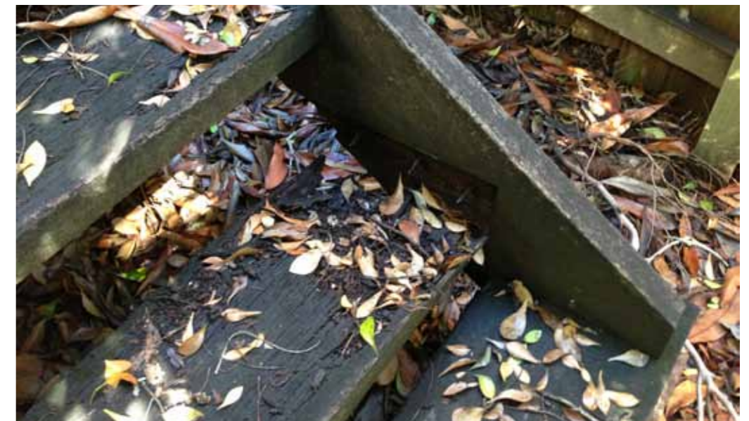
Timber stairs rotting.
