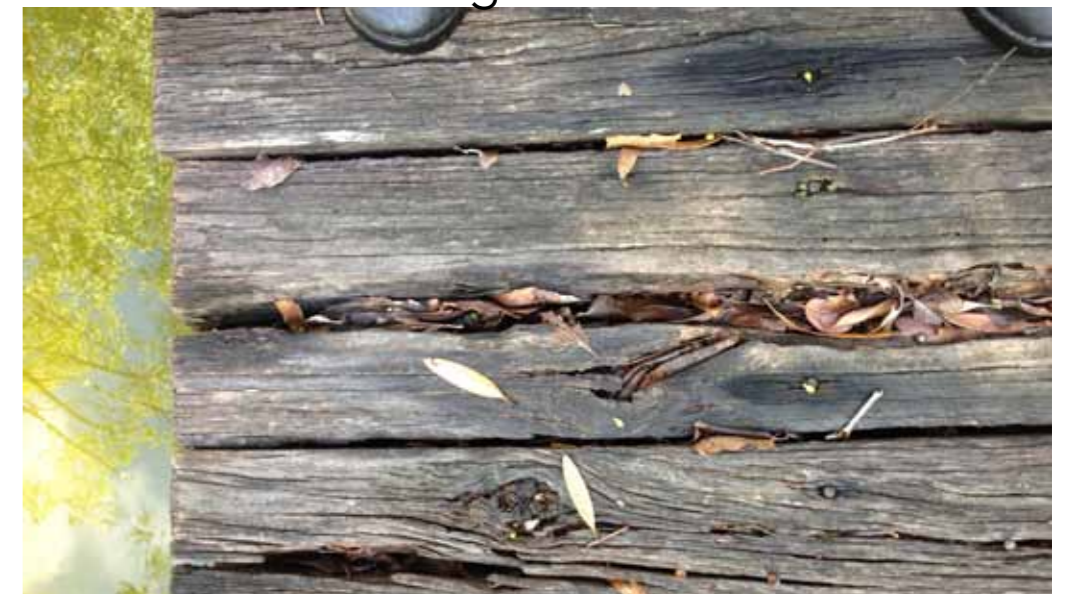
Rotted timber pool surround (200x75 CCA treated HWD double nailed & split down the middle)
