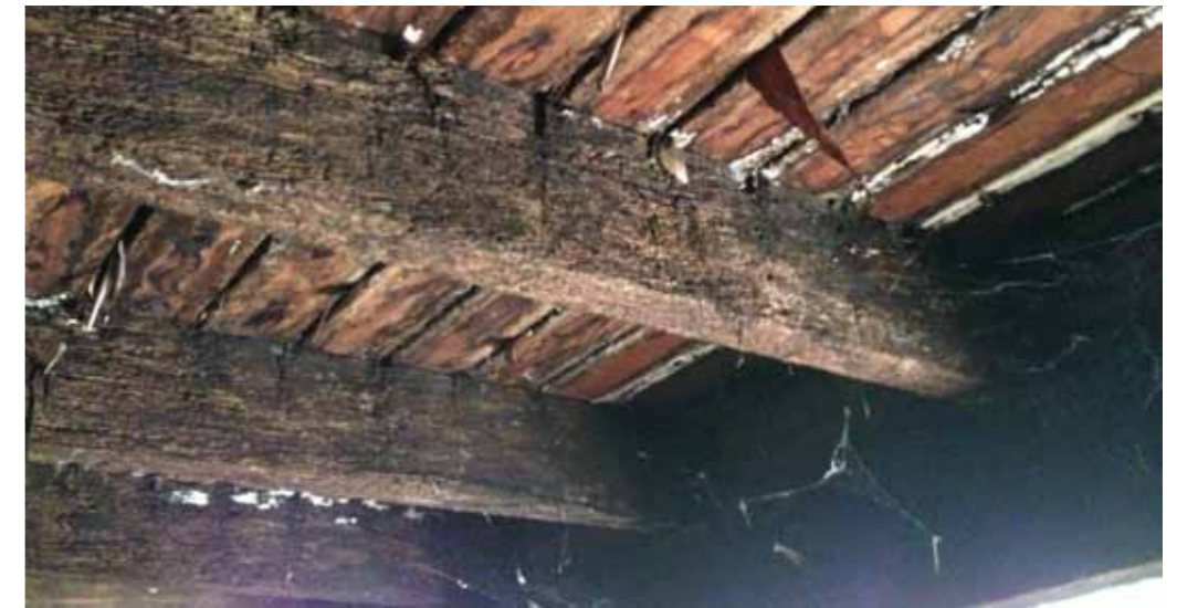
Underside of a verandah that is failing.
