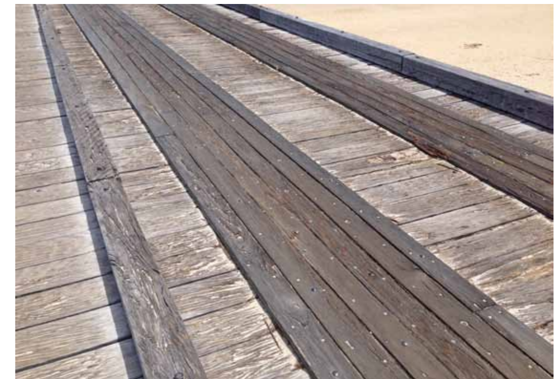
KFBRV Jetty - Satinay piles -The vehicle track boards are starting to fail - Natural weathering / no treatment
